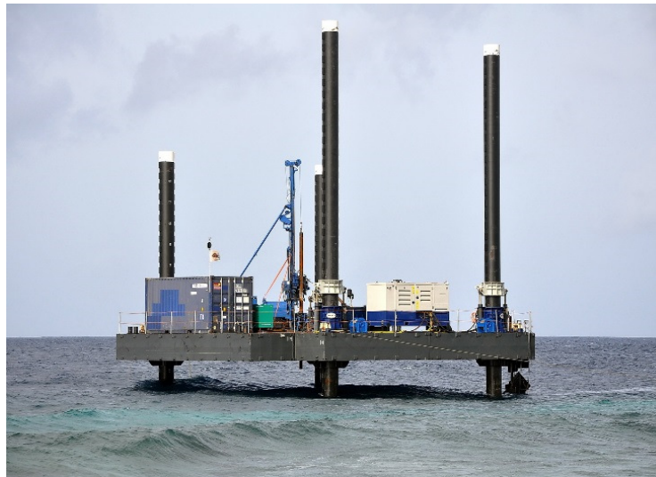
Figure 2: Jack up barge capable of adjusting to tides to enable the construction of the piers and pilling activities.
