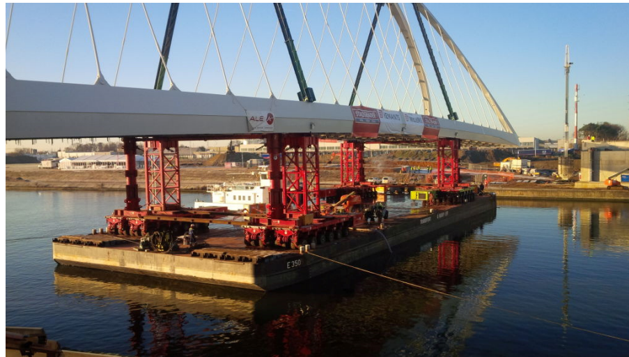
Figure 5: Bridge deck jacking from barge to reduce the need for large temporary work jetties and cranes
